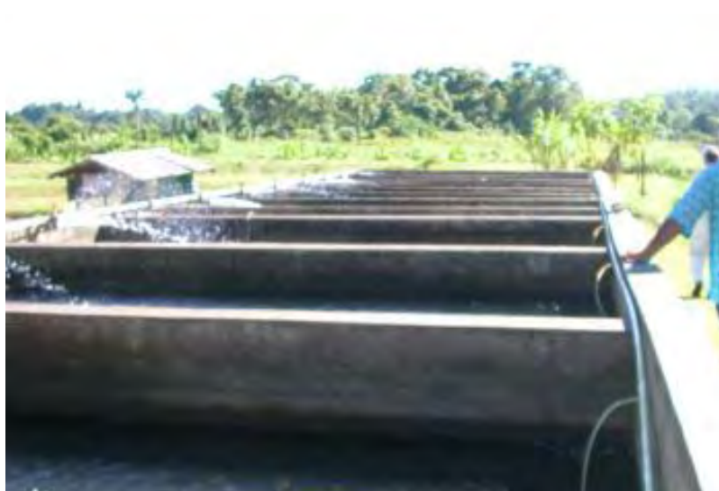
Figure 11. Concrete culture tanks at the Ministry of Fisheries and Forestry Aquaculture Center Naduruloulou, Fiji.
